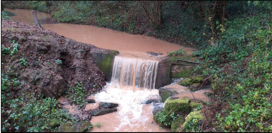
Figure 11: One of the many small storage areas installed as part of the Worcestershire Natural Flood Management pilot project, which was funded by Defra over the last 3 years
