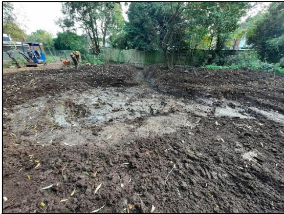
Figure 5: A recently completed pond with a leaky dam that aims to 'slow the flow' to the benefit of local drainage systems in Hollywood (this is scheme C5 in Table 1)
