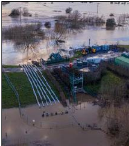
Figure 1: Kempsey pumps in operation in January 2021
